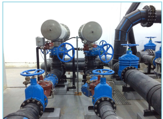
Supply & Installation of HDPE & PVC pipes and fittings Sulaibiya Wastewater Treatment Plant (Client: ABJ Engineering & Contracting Co. – Division of Kharafi National)
