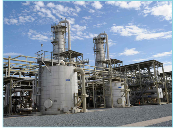
Joint Operations (Chevron) at Wafra Installation of HDPE pipeline (Client: Gulf Combined Est. – KSA)
